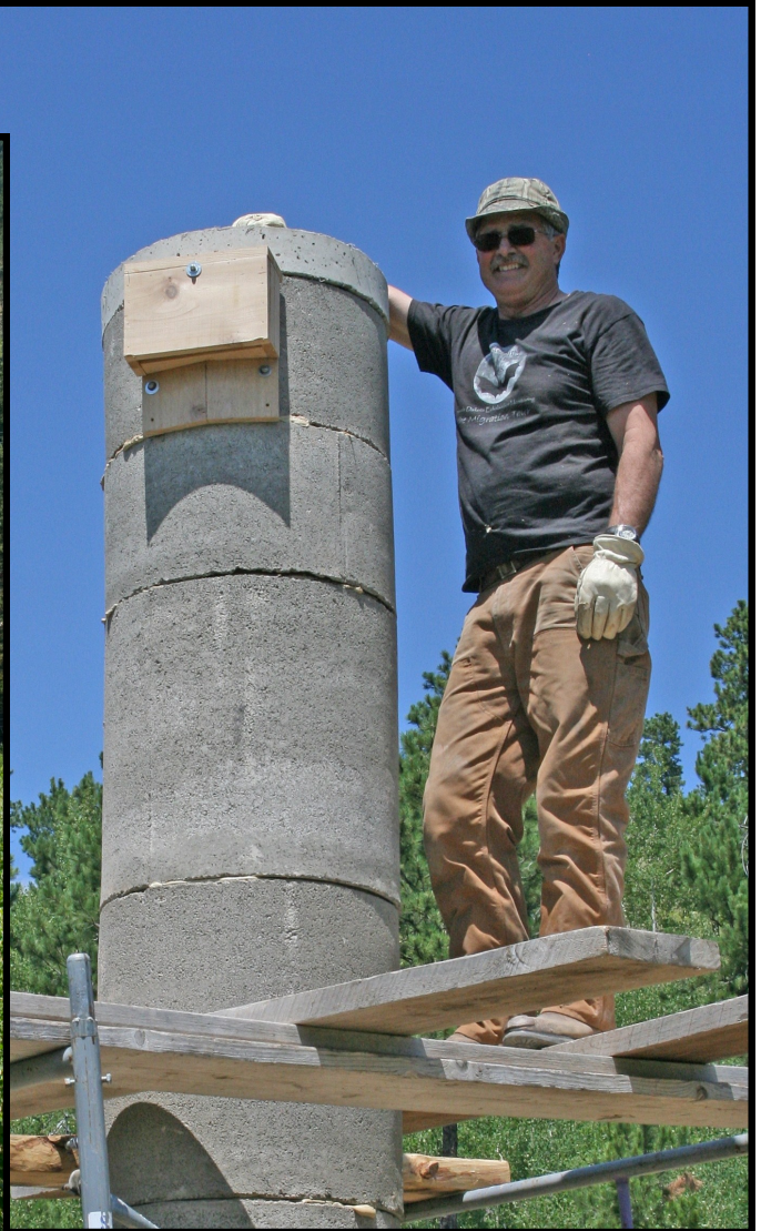
Paul Schipke takes a break once the concrete lid is in place on top of the structure.
